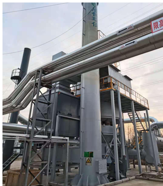
厂区现有 RTO 焚烧炉
